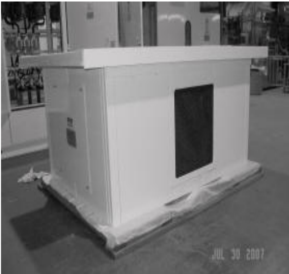
Enclosure for Generator Neutral Reactor Figure 3
