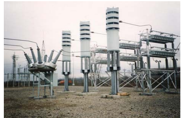
138 kV, 62 Mvar, 5 th Harmonic, Open Air Filter Bank
