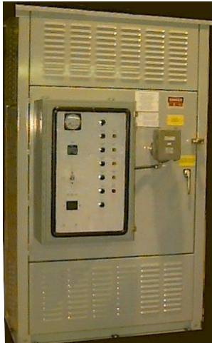
480 Volt, 400 kvar, 5 th Harmonic Metal-Enclosed Filter Assembly
