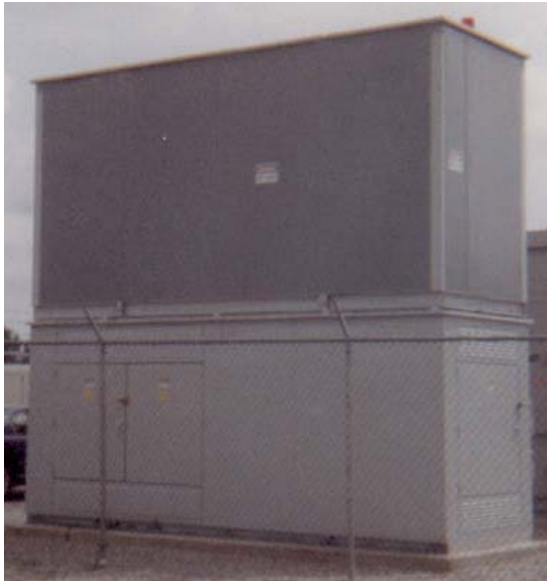
25 kV, 3 Mvar, 4 th Harmonic Filter Bank With Enclosed Air Core Reactor
