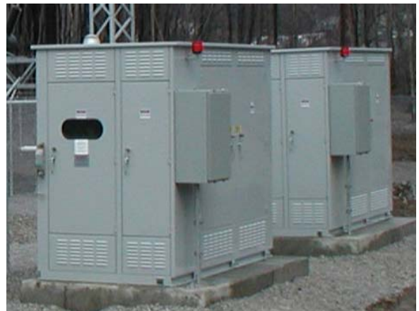
12.47 kV, 4 th Harmonic Filter Banks – Each with Two 1200 kvar Steps
