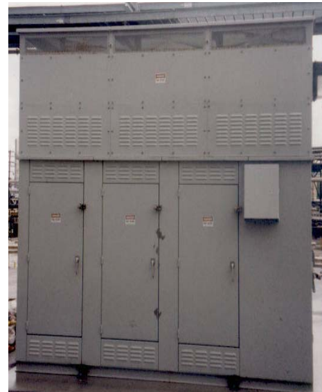
13.8 kV, 3.5 Mvar, 11 th Harmonic High-Pass Filter Bank with Enclosed Resistor on Top
