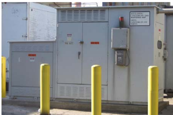
Conversion of 4.16 kV, 1200 kvar Capacitor Bank to 1900 kvar, 4 th Harmonic Filter Bank
